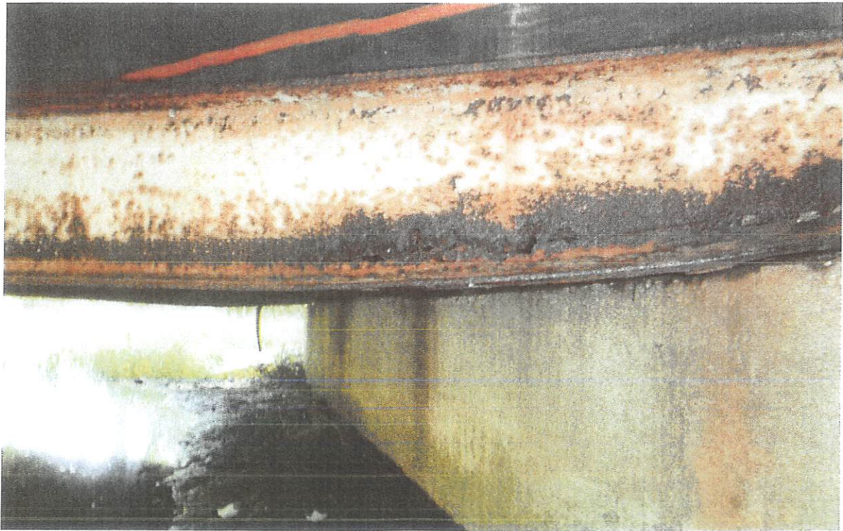
Photograph 3 - Slotted holes along web of interior girder (B4) and significant sagging. Girder located under wheel path.
