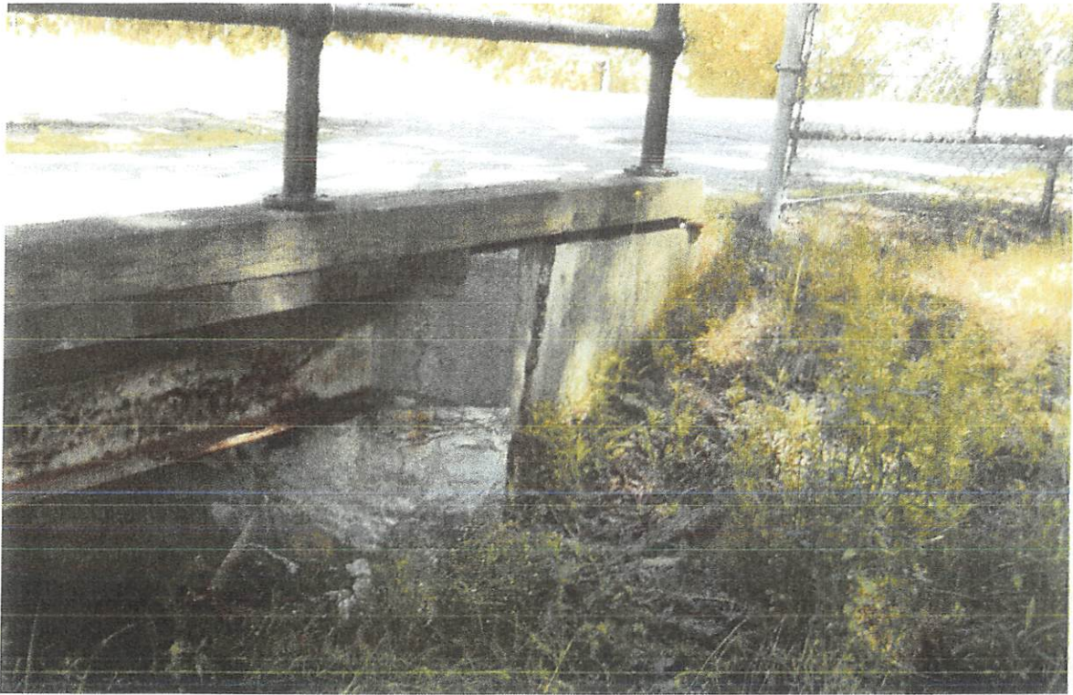
Photograph 6 - Cracked northwest wingwall, separated from abutment
