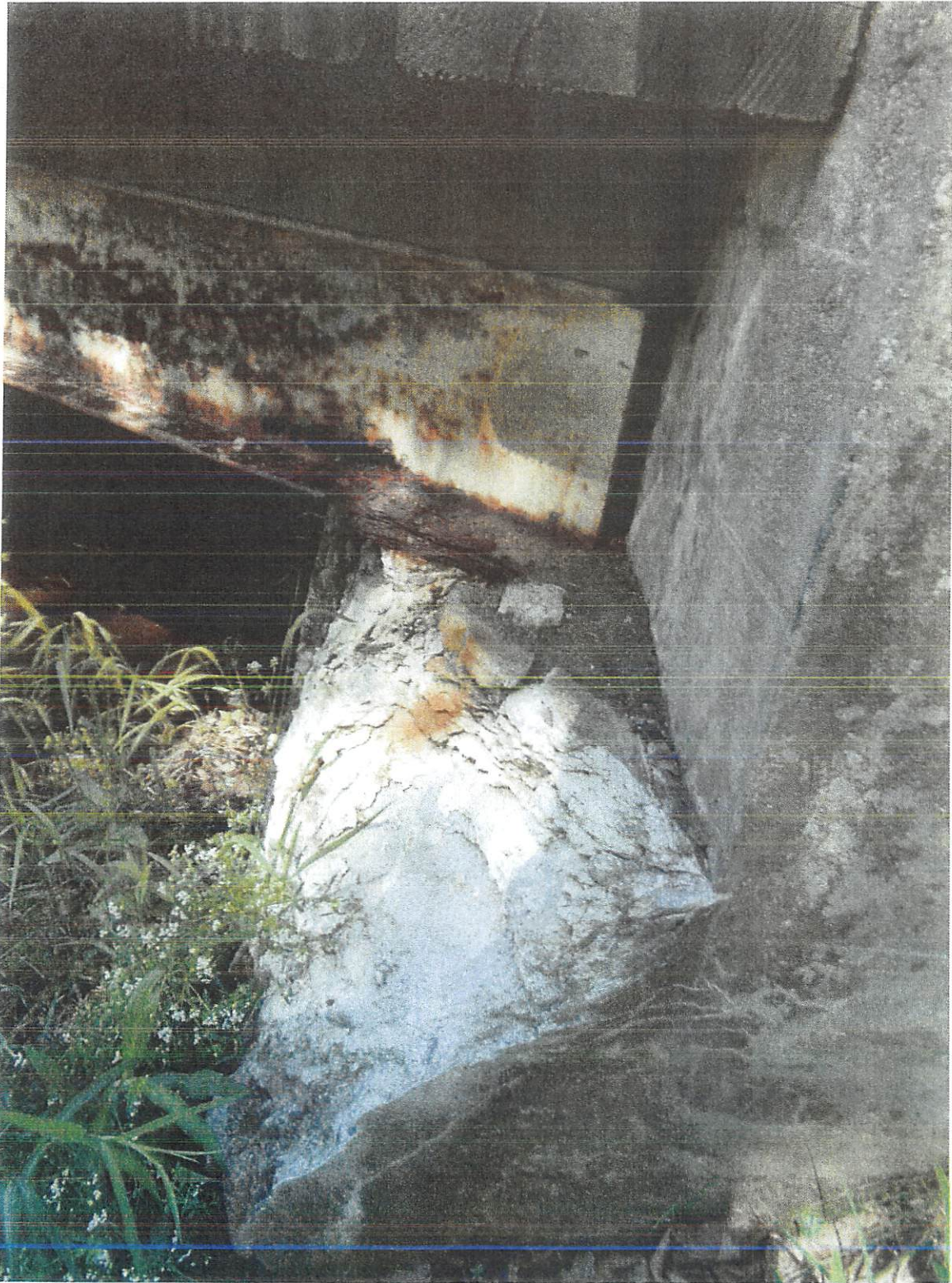
Photograph 4 - Spalling and delaminated concrete at North Abutment, hole in web of Easterly fascia girder (B1). Debris collected on abutment seat.
