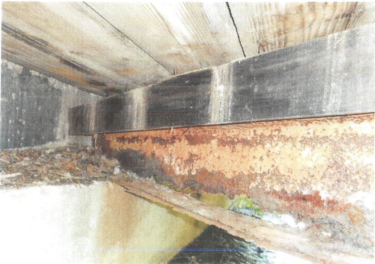
Photograph 1 – Interior girder failed due to crushing and large slotted hole in web. Note the 3" to 4" separation between the timber blocking and the timber decking. Girder located under wheel path.
